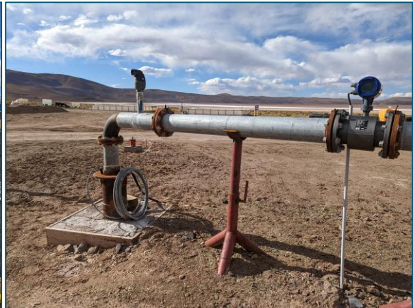
Figure 30: Pumping station (Pata Pila licence)
